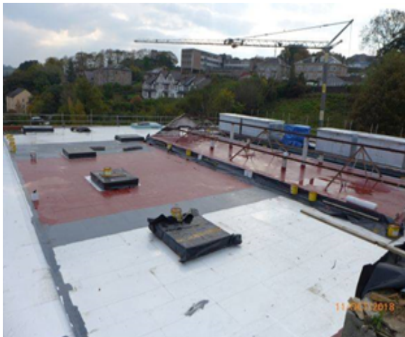
Looking South: Roof Over Auditorium/Main Hall General View (NB: Exposed Roof Trusses to Auditorium Roof Light & Ventilation Plant).
