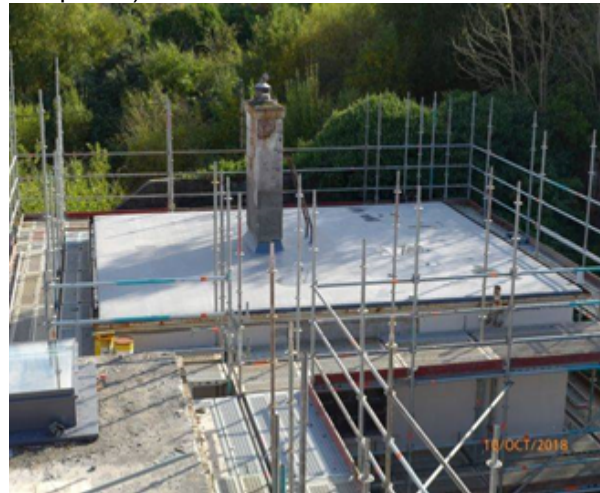
Looking South: General View of Caretakers House Roof (NB: gutters yet to be replaced).
