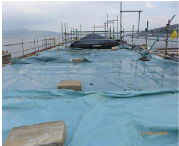
Looking East (facing Argyle St): Roof over Fly Tower/Stage Area (NB: Temporary waterproof protection).
