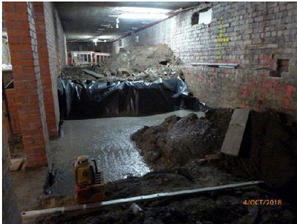
Auditorium Undercroft Area: (NB: Work in Progress: new concrete floor slab insitu for creation of new Staff/Utility/stair area).
