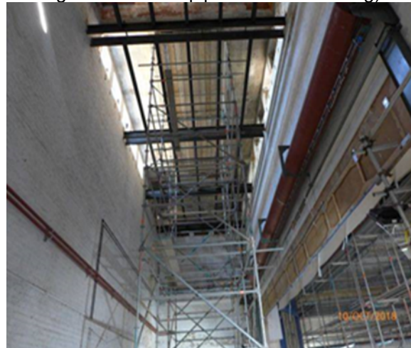
Stage Area: General View of Scaffold (Crash Deck) below existing roof light.
