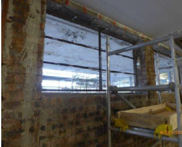
Exhibition Space (East Elevation – Argyle St.): Removal of existing external windows and installation of new Crittall windows.
