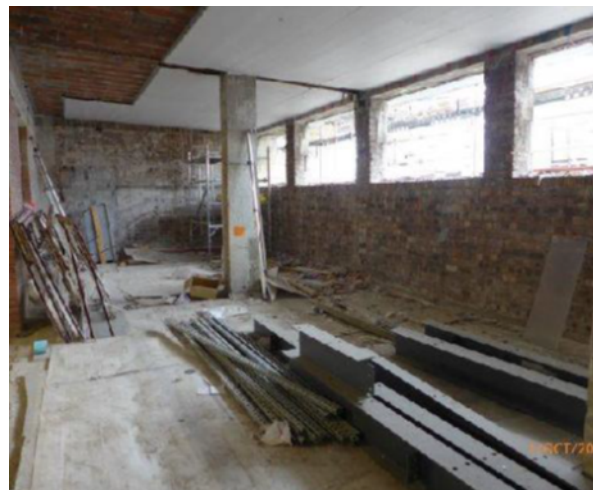
Exhibition Space (East Elevation – Argyle St.): Removal of existing external windows and installation of new Crittall windows.
