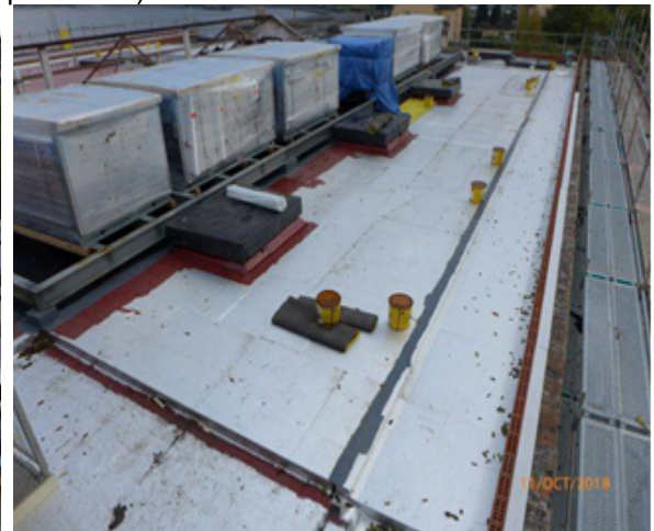
Looking South: Roof Over Auditorium/Main Hall along the West Gutter - General view (NB: Ventilation Plant insitu).
